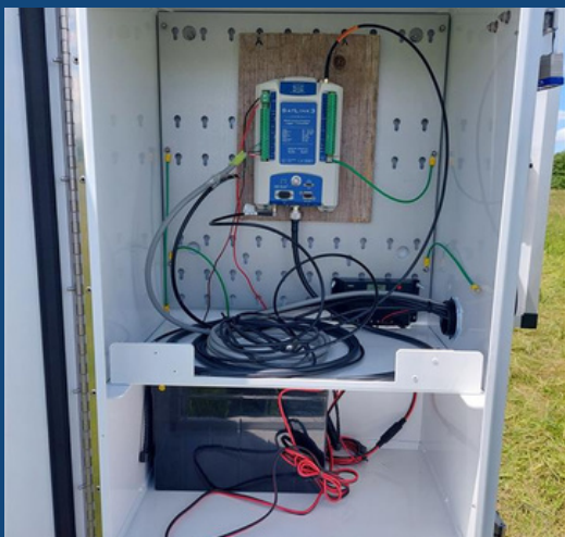
Monitoring equipment inside the weather station.
