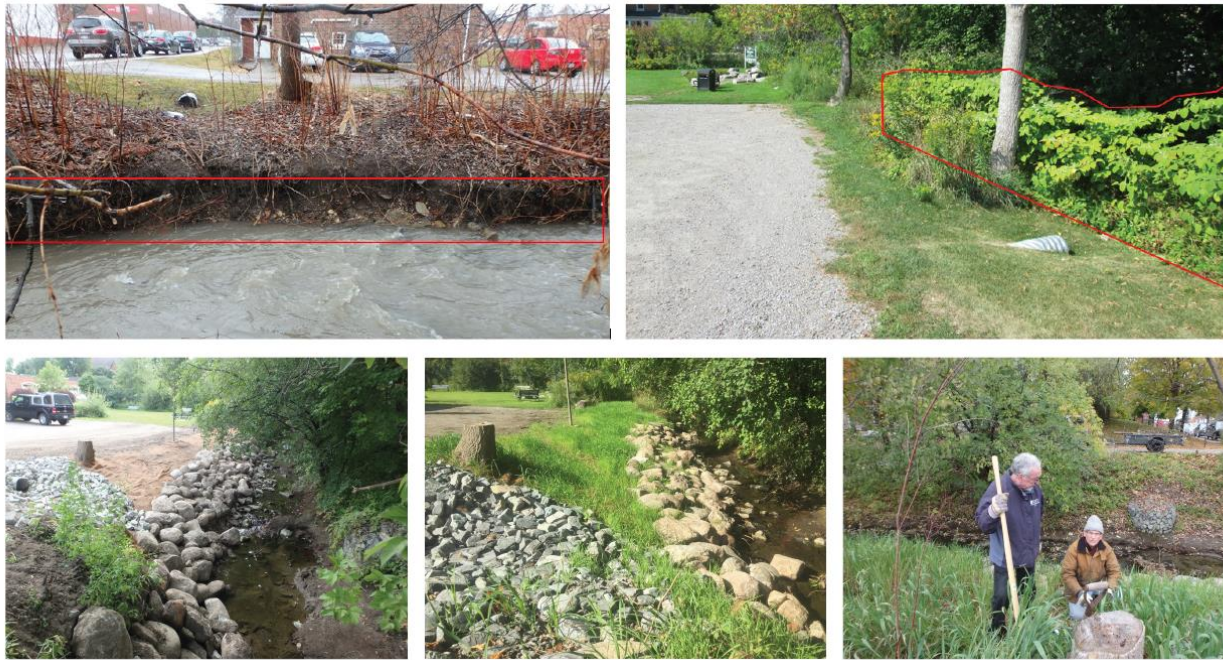
Figure 6 The series of photos above shows the progression of a "shovel in ground" project conducted as a part of an Urban Stewardship program. The project addressed issues of shoreline erosion (top left), and an infestation of invasive Japanese knotweed (top right). A restoration construction project followed by a community planting restored this stretch of shoreline in Port Perry to a more natural and functional state.
