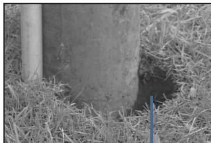
Faulty annular seal
